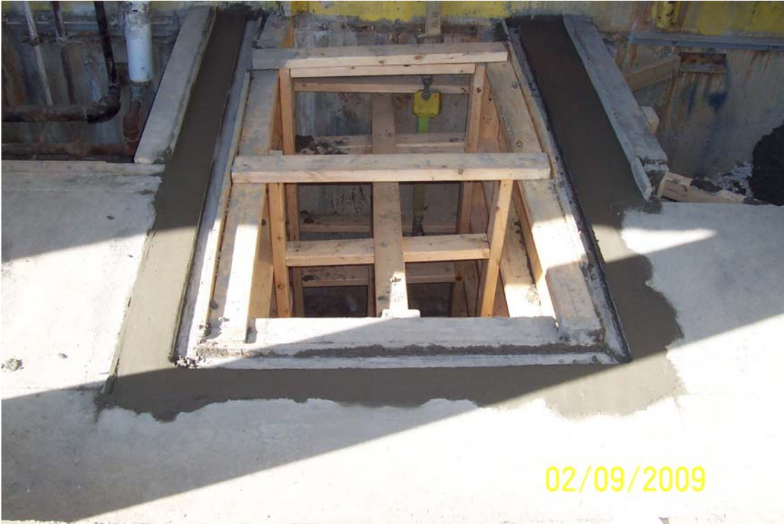
Photo 23 - Sump excavation looking west—wooden forms installed and concrete sump walls were poured.
