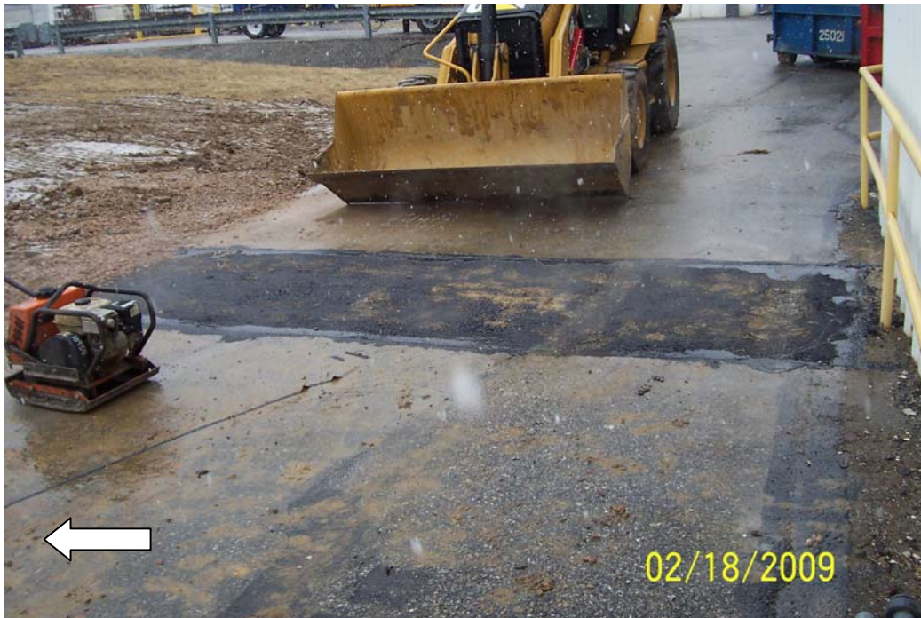
Photo 28 - Building 41 outside pipe trench asphalt surface completion. North indicated by white arrow.
