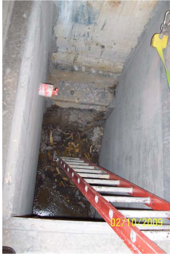
Photo 24 - Sump looking west-wooden frames were removed, liquid in bottom of sump pit. 4" dia. perforated PVC pipe entering sump with compression cap.
