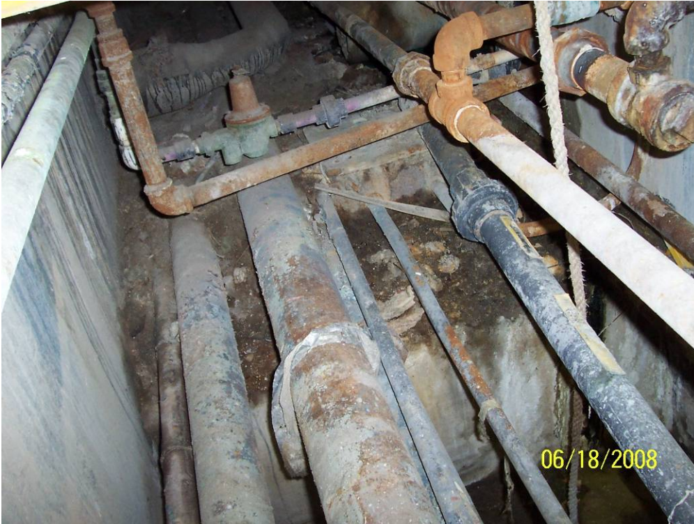
Photo 5 – View of pipe trench looking south from the deeper segment, near SWMU 40.
