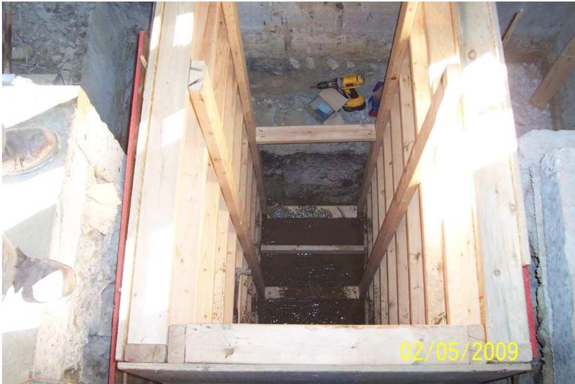
Photo 21 - Sump excavation looking west—wooden forms being installed, concrete bottom of sump with 2” of liquid in bottom of sump.
