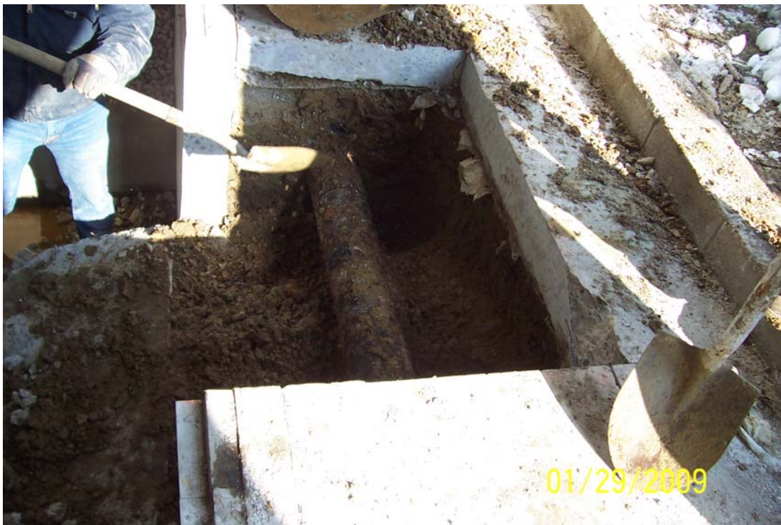
Photo 12 - Building 41 sump excavation. Interior 6" dia. metal pipe that took a 90 degree turn and re-entered pipe trench in front of EQ tank. Pipe was cut and plugged with concrete.
