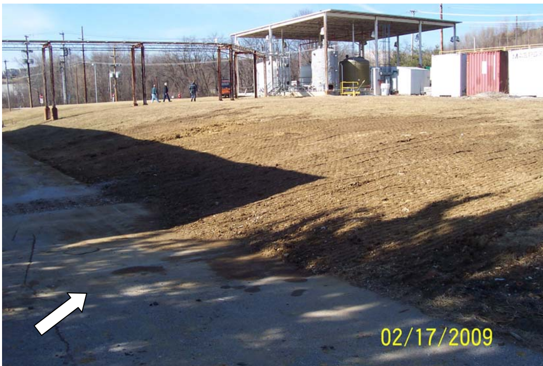
Photo 29 - Building 41 vault and test pits backfilled and returned to grade. North indicated by white arrow.
