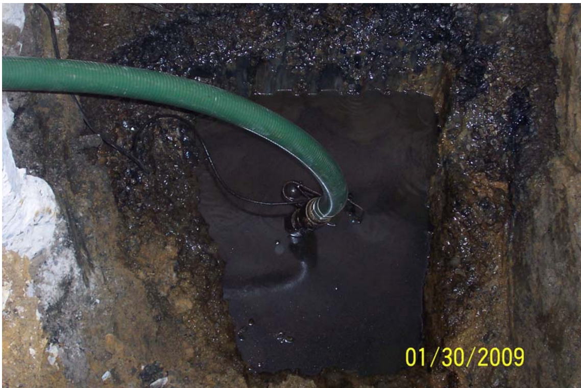
Photo 18 - Sump pump used to remove liquid from sump excavation. Liquid was placed in a tote for storage until it was transferred off-site.
