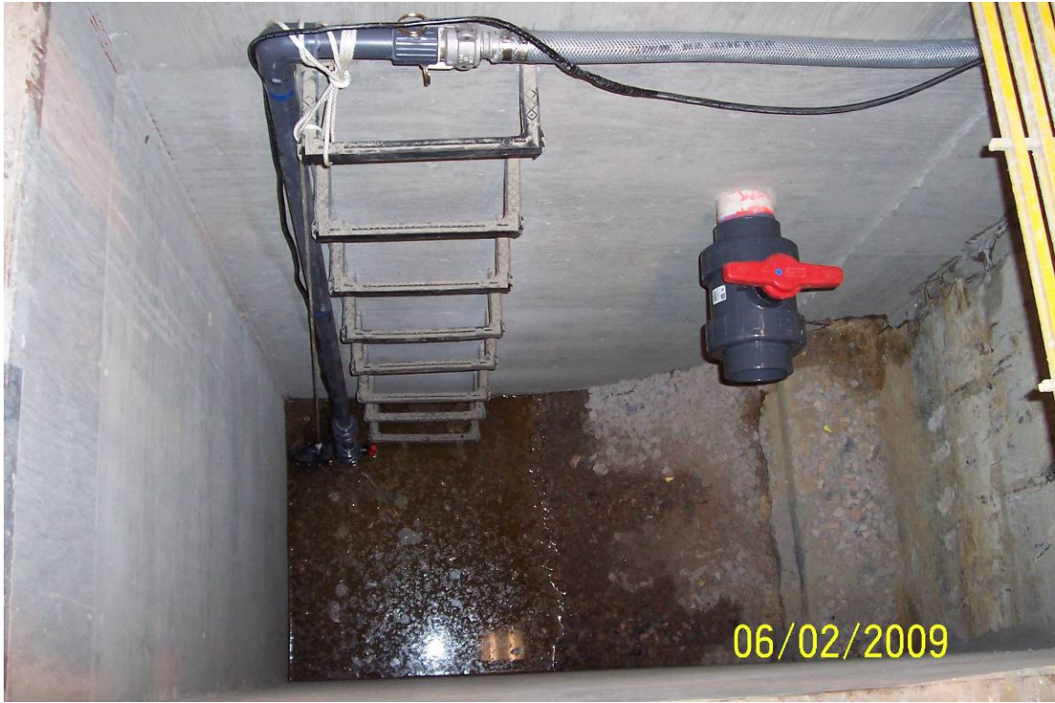
Photo 30 - Pump installed in sump and new valve placed on pipe connection from south trench.
