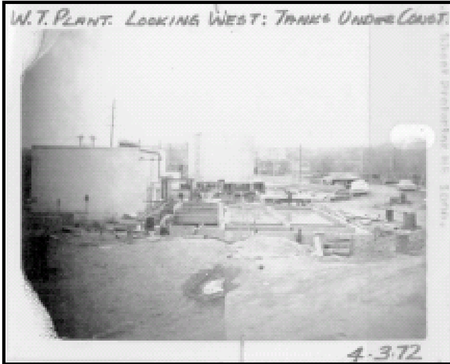
Photo 13 – April 3, 1972 photo. View looking west, east of new WW tanks for Bldg 41. Apparent sump/cover at northeast corner of WWTP building.
