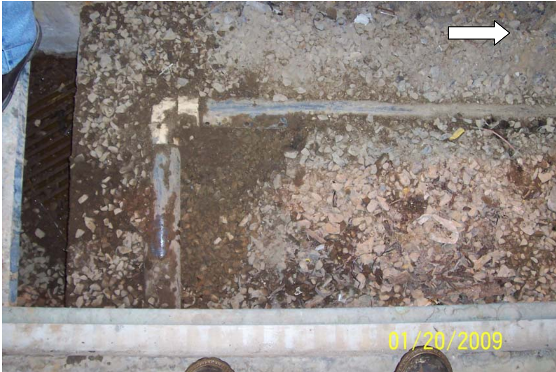
Photo 7 - Building 41 interior trench – 4” PVC undocumented pipe. Note perforated pipe running N-S in trench. The pipe was solid running E-W. North indicated by white arrow.
