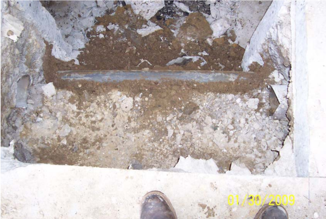
Photo 13 - 4" dia. undocumented PVC pipe located under a 6" dia. pipe found in the pipe trench that was excavated during sump excavation. 6" pipe has already been removed in photo.
