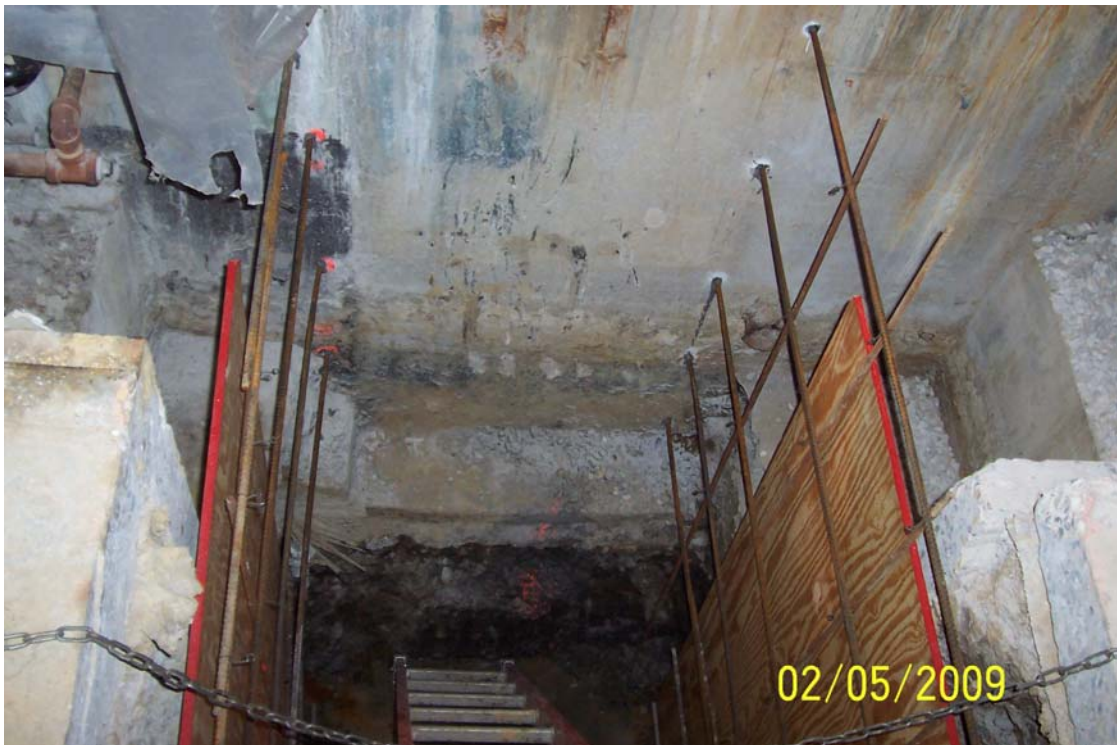
Photo 20 - Sump excavation looking west—rebar cage anchored into settling basin wall and plywood shoring of sump walls.
