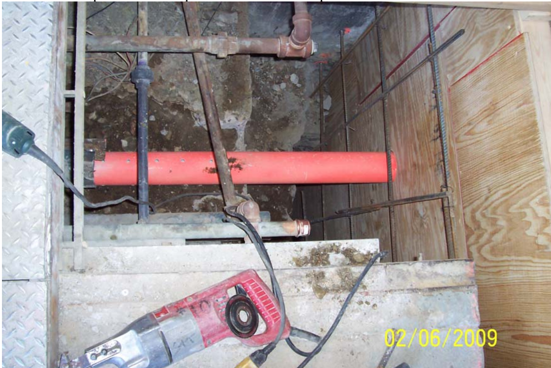
Photo 22 - 4” dia. PVC pipe installed with perforation from pipe trench in front of EQ tank into sump.
