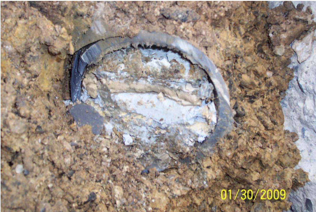
Photo 14 - 4" dia. PVC pipe was filled with a white flaky substance that was sampled and presumed to be an alkaline wastewater treatment agent.
