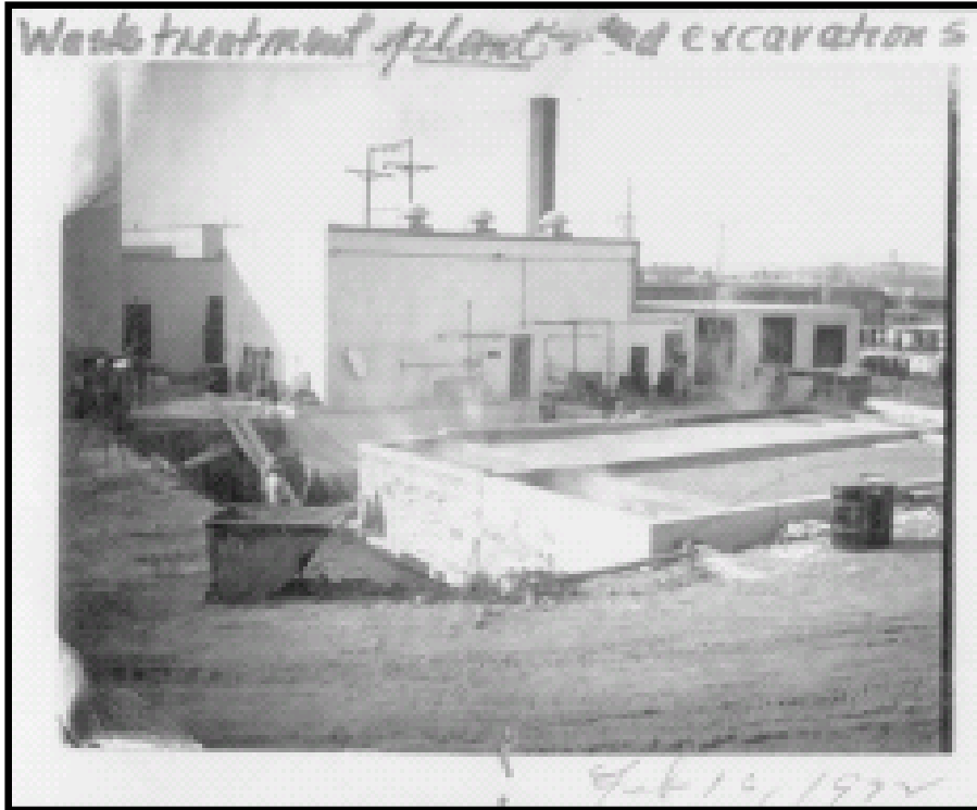
Photo 9 – February 1972 photo. View looking southwest from northeast corner of new Settling tanks. Note western WWTP building extension.
