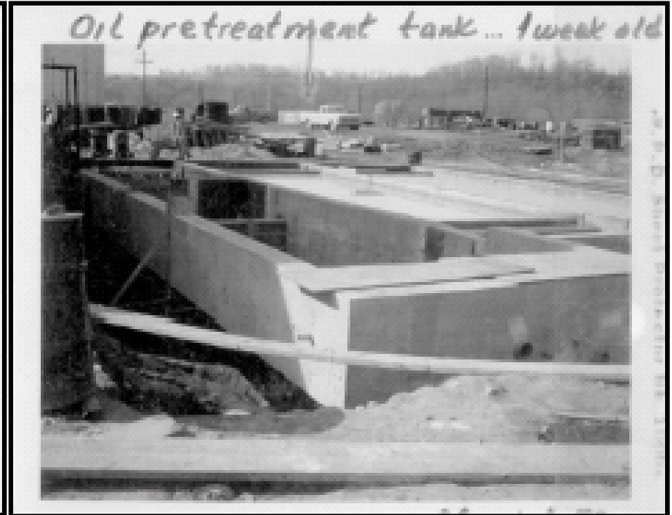
Photo 10 - March 1, 1972 photo. View looking west from east side of new EQ tank (inside of south settling tank appears to be asphalt coated).
