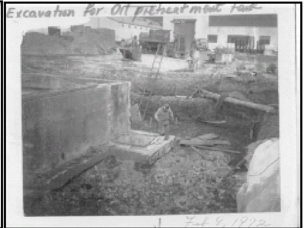
Photo 6 - February 9, 1972 photo. View looking northeast from near north mandoor of WWTP building. Note former sump pad and excavation for new EQ tank.
