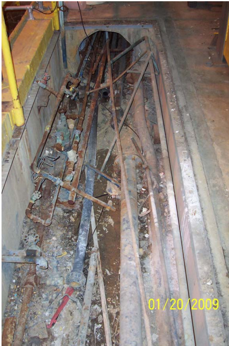
Photo 4 - Inside Building 41 pipe trench before pipes were removed. View looking north from the EQ Tank.
