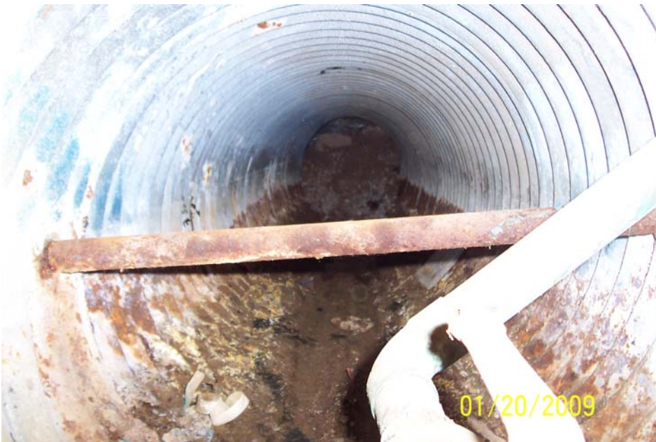
Photo 6 - Looking north into 24" dia. corrugated pipe that connected interior and exterior trench under Bldg 41. Pipes were removed and exterior trench was backfilled with crushed stone.
