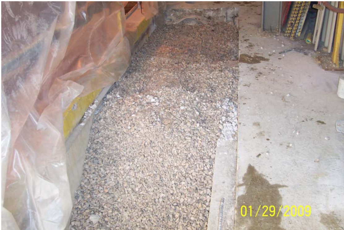
Photo 11 - Building 41 interior pipe trench backfilled with crushed stone after samples were collected.
