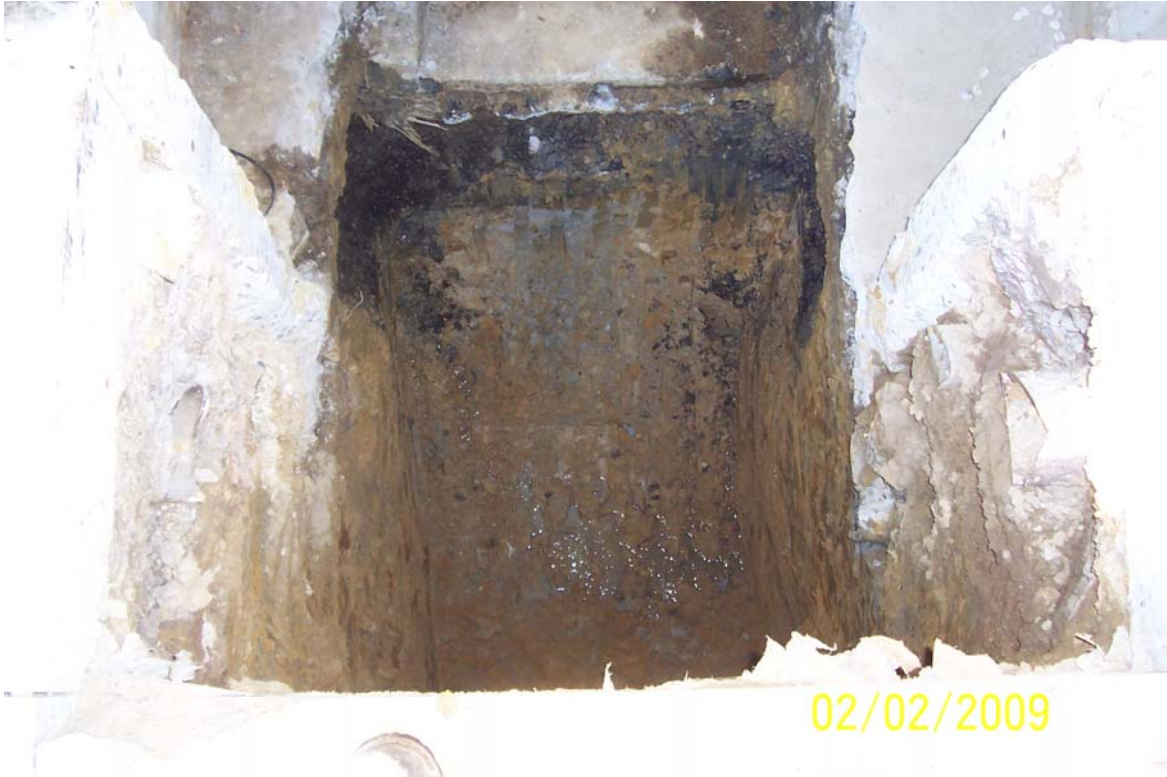
Photo 19 - Sump excavation. Impacted soil visible and liquid entering sump from impacted gravel zone. View looking west.
