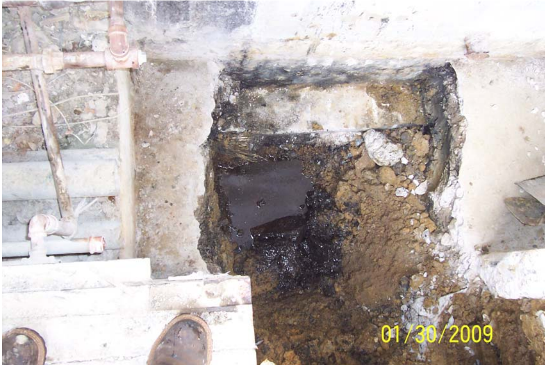
Photo 17 - Black liquid entering sump excavation from under south settling basin footer.
